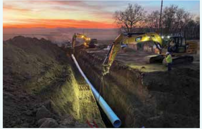
NRWA Grand Prize photo taken by Banner's Nick Fuhr of pipeline construction between Beresford and the Big Sioux River
