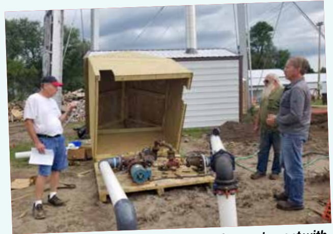
Inspecting Tulare's temporary pumping equipment with Board Chairman Brian Hull, City maintenance worker Archie Stanley, and Calvin Kindle from Mid-Dakota Rural Water System.
