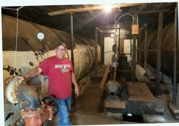
SDARWS Circuit Rider Greg Gross took this picture in Hudson where he got a look at these water storage and pressure tanks from the beginning of the century that are still in use today.
