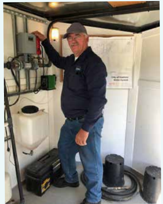
SDARWS Circuit Rider Nick Jackson in Kadoka assisting with leak detection and flow/pressure testing.
