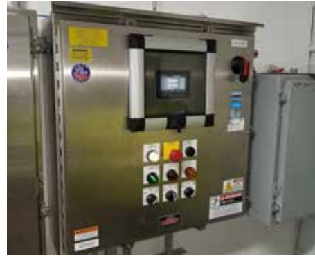
Screen control panel
