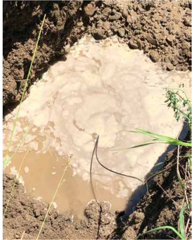
Saturation in the ground at two feet down
