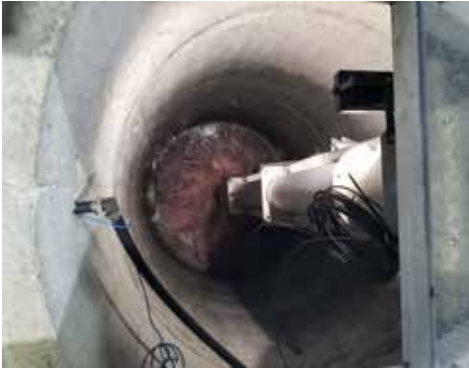
Screen wet well
