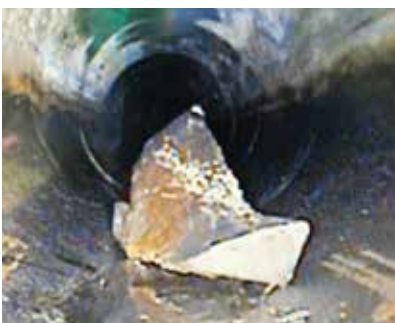
Camera shot of a rock stuck in the pipe
