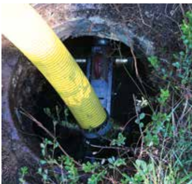
Camera set in an access point and ready to work.
