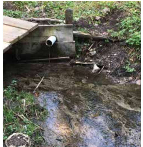
All of the springs converging and heading into the collection pipe.
