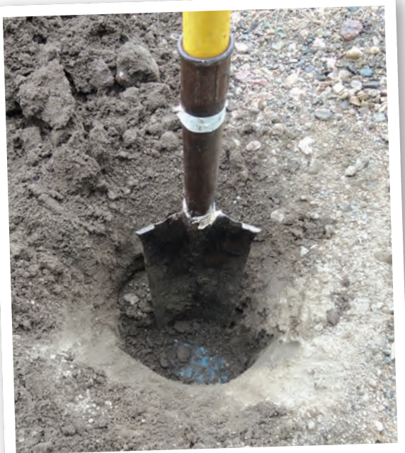
Curb stops aren't always at ground level...
