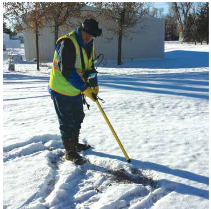
The largest leak in Vale was found on a main down an alleyway.
