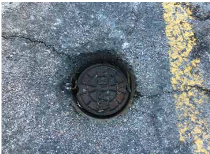
Before picture of a riser that was too low.
