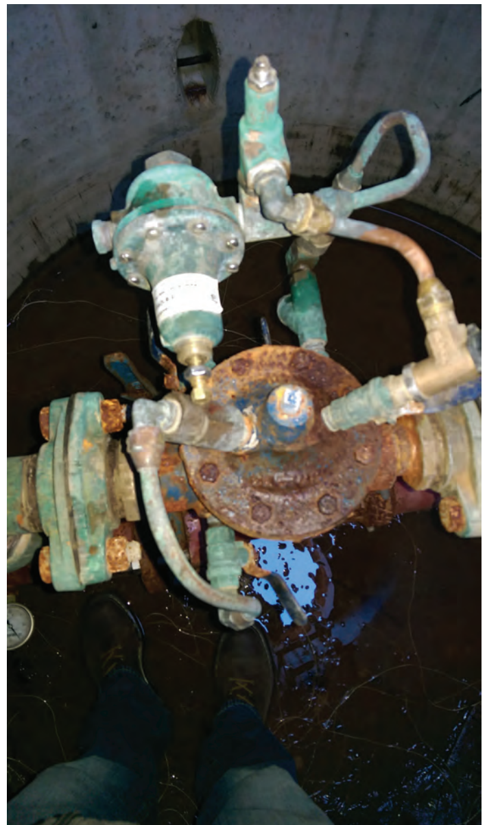
Control valve that needed complete teardown and cleaning
