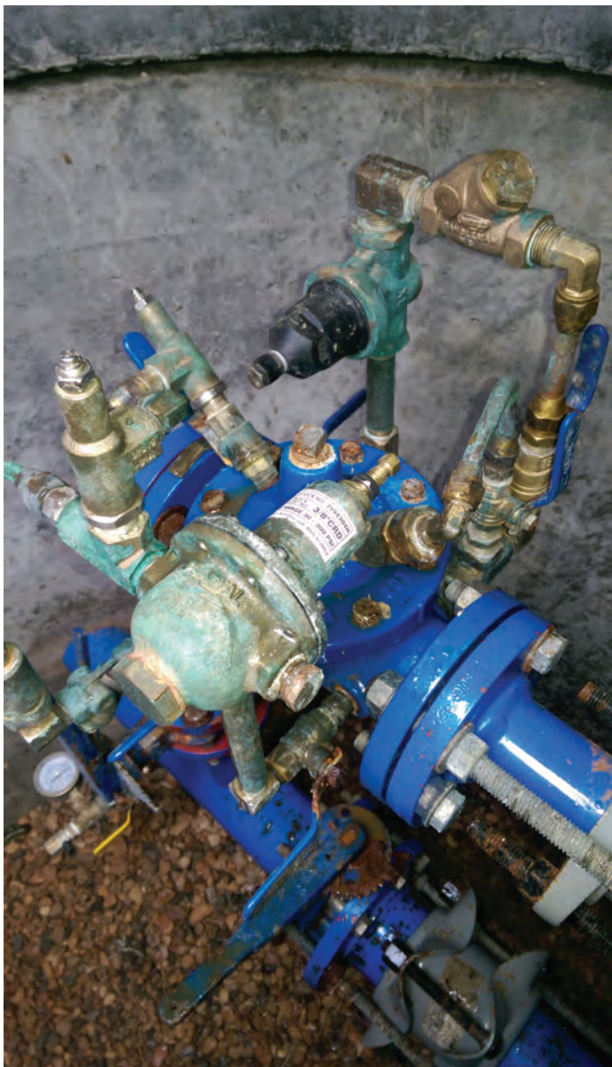
Control valve that needed the speed controls cleaned and exercised for proper operation.
