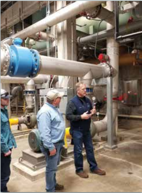
Some of the SDARWS staff stopped by the Mid-Dakota water treatment facility for a tour while in Pierre before the ATC.
