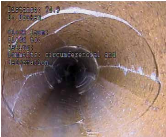
Sewer main – repair or replace?
