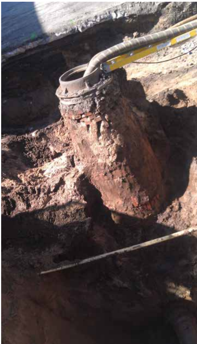
Brick manhole partially collapsed on a sewer main. Repair or replace?
