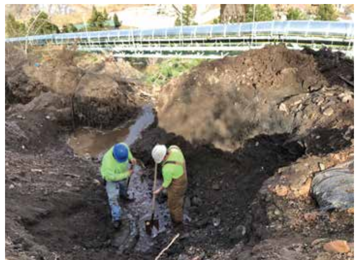
Inspecting the leak on the fittings.
