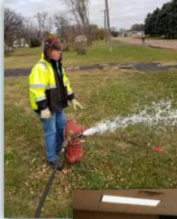
SDARWS Circuit Rider Greg Jeff Fossum assisting with flushing hydrants, pressure testing, and leak detection in Egan.
