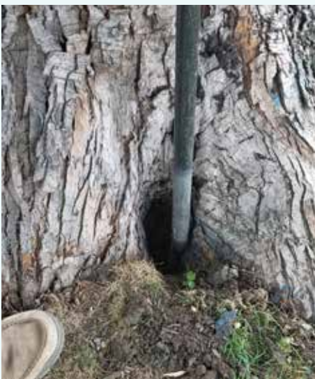
Locating curb stops can be a challenge... our Circuit Rider Jeff Fossum found this one under a tree while mapping a system!
