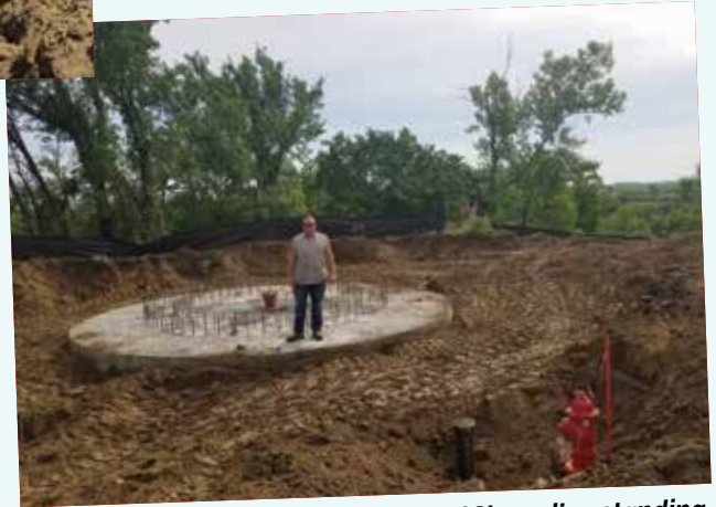
Monstrose city water operator Daryl Sieverding standing on the base of the city's new water storage tank.
