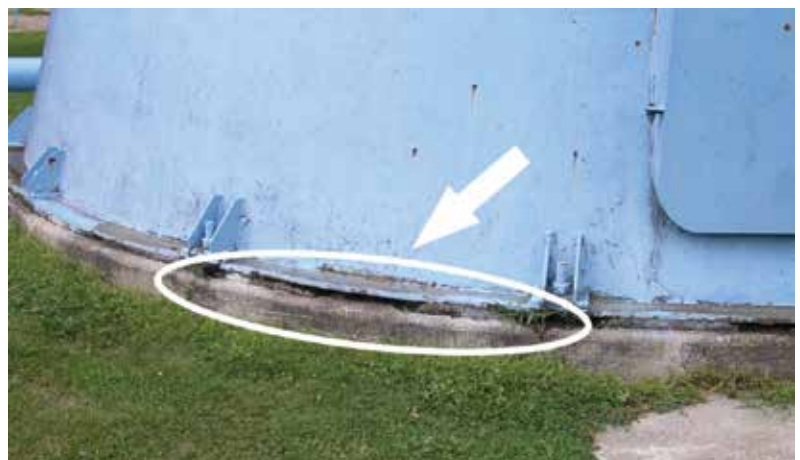
Improper and failed grout between the foundation and the tank base plate.
