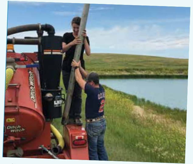
SDARWS Wastewater tech Abbey Larson and Utilities Manager Frankie Ducheneaux were cleaning valve risers and exercising valves at the lagoon site in Isabel.
