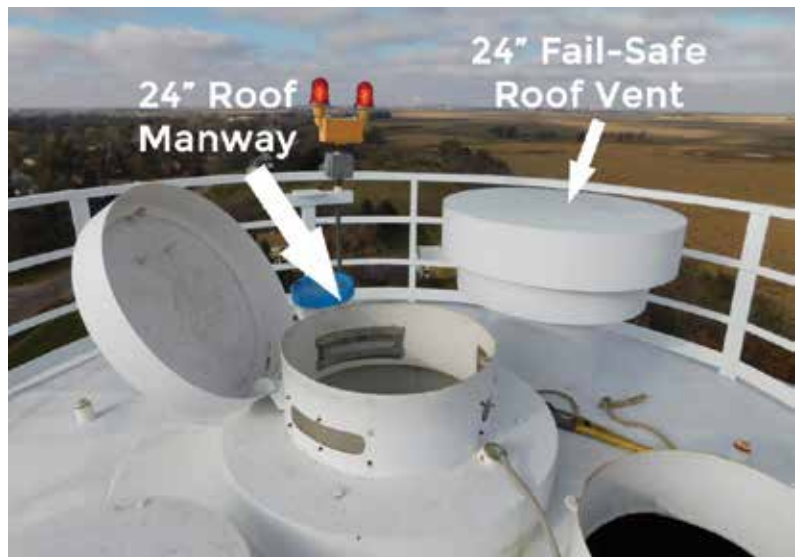
These are examples of a proper welded steel vent and manway that meet OSHA and AWWA standards.
