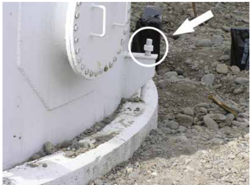
Anchor bolts improperly secured can cause structural issues.
