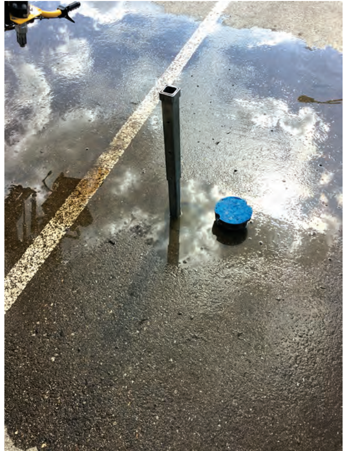
Packing bolts rotted away and valve leaks when not in the full open position.
