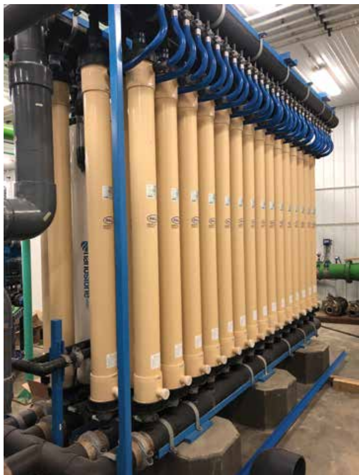
The last filtration skid is to be rebuilt and fitted with Nanostone ceramic filter elements
