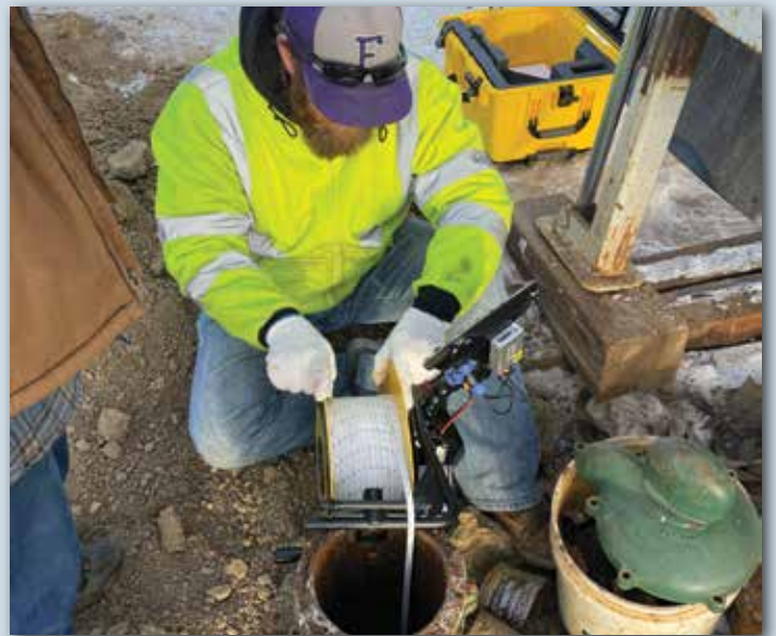
Source Water Protection Specialist Kevin Christenson inspecting the well casing with a bore camera in Hermosa.
