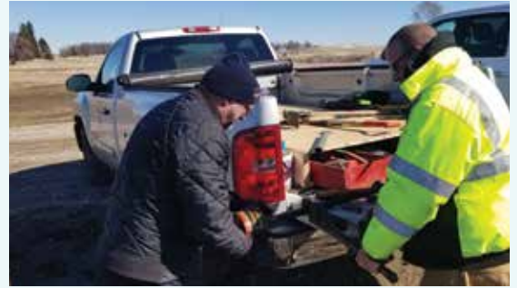
SDARWS Circuit Rider assists Valley Springs Operations Specialist Blane Eilts with hydrant repairs.
