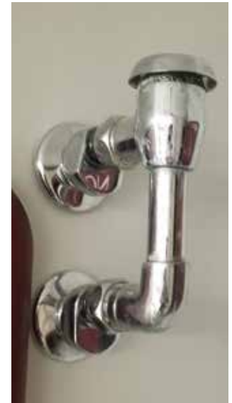
Air Vacuum Breaker (AVB)
