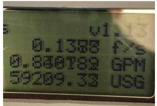
Chlorine being pumped from the leak detection trailer to the injection point.
