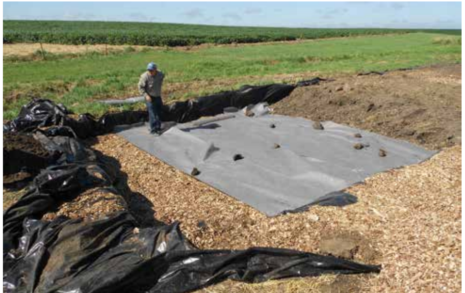
Bioreactor filled with woodchips, geotextile is being laid on top and topsoil is being backfilled onto geotextile. Image by Chris Hay.
