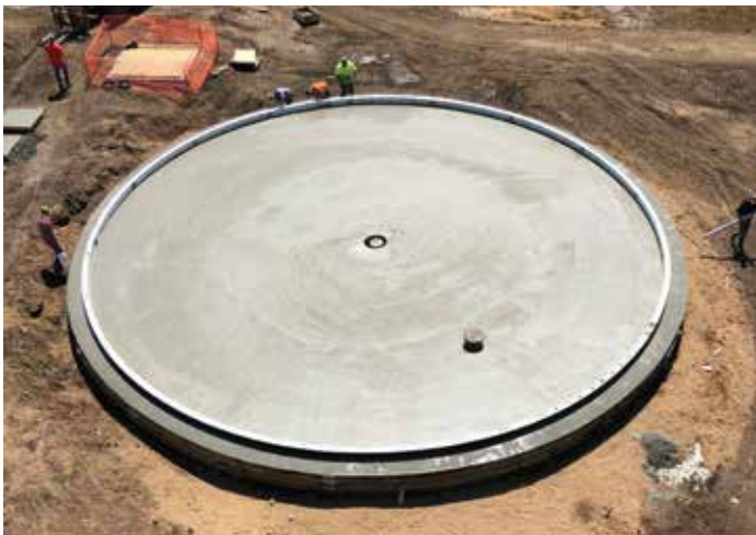
Pouring concrete floor slab for recently completed 600,000 gallon glass lined storage tank at the 1.6 million gallons per day (gpd) DeSmet treatment plant.
