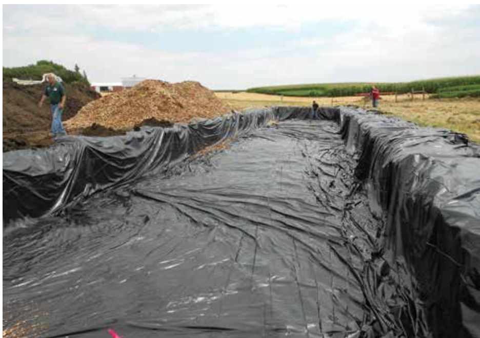
Bioreactor dug, lined, and ready to be filled with woodchips. Image by Chris Hay.
