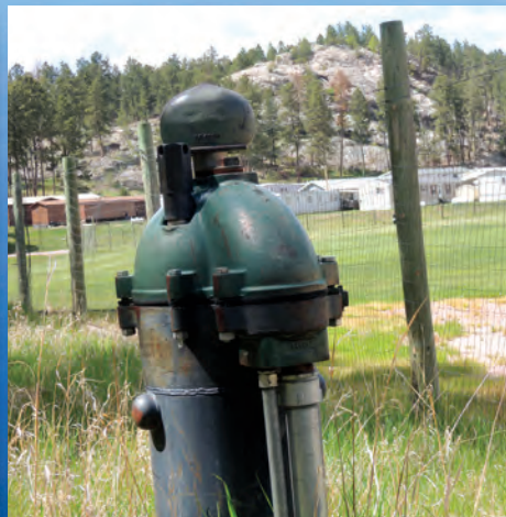
City of Custer well in fractured granite.
